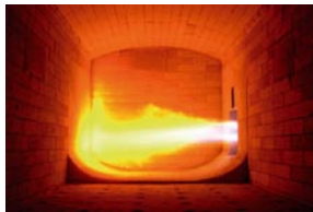
EBF – Injection burner with stoker auger
