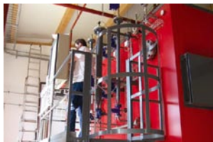
Steam dome of an 840 kW boiler
